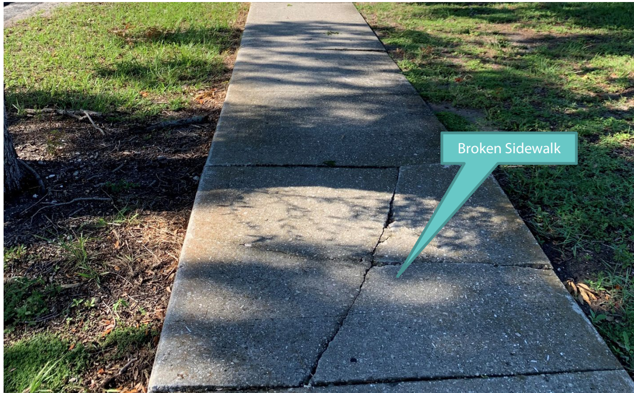
Figure 27: Broken Sidewalk near Cortez Commons (looking south)
