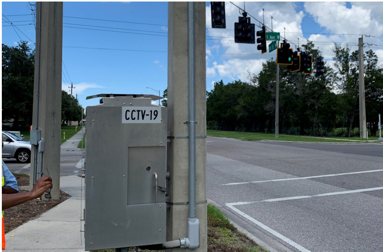
Figure 13: Closed Circuit Television Cabinet (looking north)
