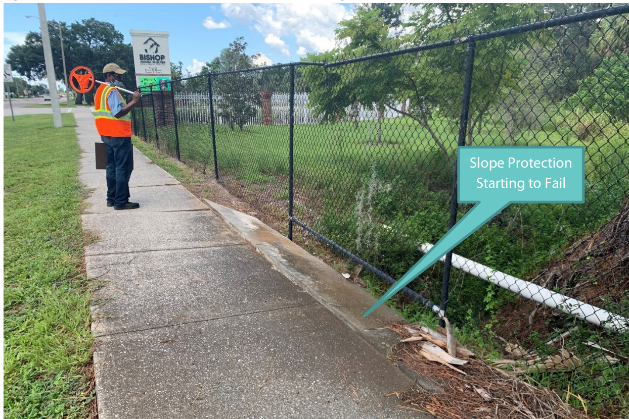
Figure 28: Erosion behind Sidewalk at Animal Shelter (looking north)
