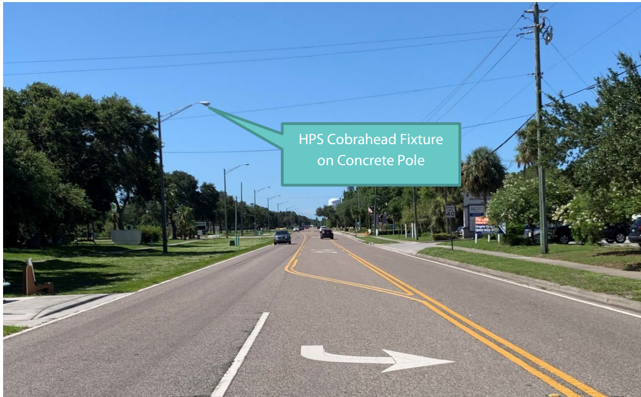
Figure 20: Lighting along 59th Street (looking south)
